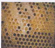
A badly scaled/fouled heat exchanger
